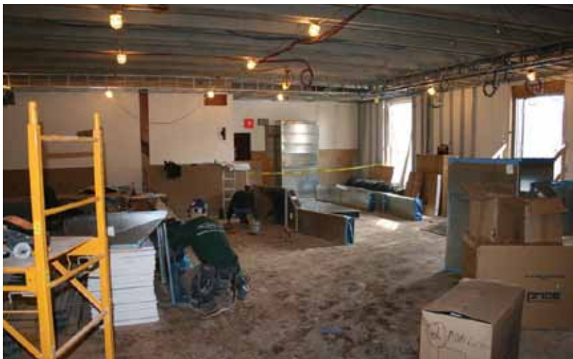
Duct work for the new HVAC system in the Fitz Henry Lane Gallery.
