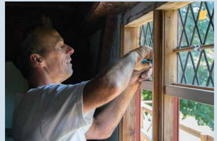
Steve Goodick of W. Herbert Goodick, Inc. makes final adjustments to the new windows at the White-Ellery House.
